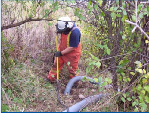
Fibre optics cable was found at proposed location for bridge foundation
