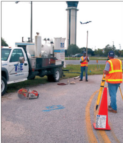
TBE Group has grown to be one of the top trenchless engineering firms in the United States, with more than 400 associates.
