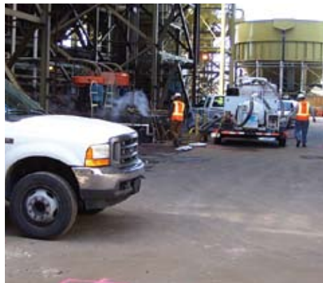
Nondestructive vacuum excavation equipment verifies the vertical and horizontal locations of underground utilities where proposed concrete support foundations will be constructed for an environmental upgrade at the Seminole Generating Station. Photo courtesy of TBE Group.
