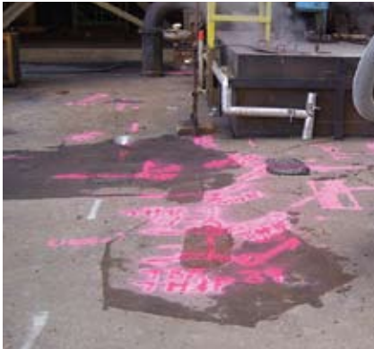
At the Seminole Generating Station Quality Level A locates are marked on the asphalt to verify the vertical and horizontal locations of the existing underground utilities and foundations. Photo courtesy of TBE Group.
